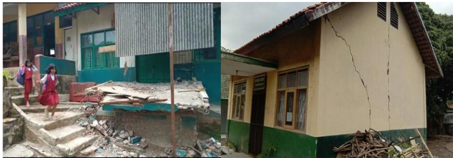
Figure 1. The damage condition of Primary School building in Bandung Regency (Source: Bandung Regency Office of Education)
