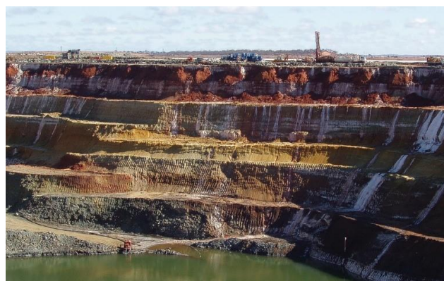
Fig 1. A gold mining GT-rig deployed on the edge of the open pit. Courtesy of Borehole Mining International, Inc. 2019
