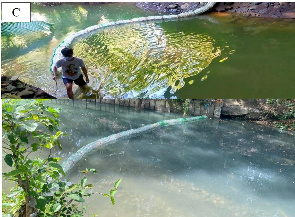
Fig. 2 Installation of river floater trash traps in (a) Gabawan River, (b) Poctoy River, and (c) Bangon River.
