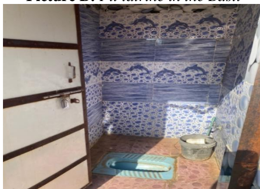
Picture B: Pit latrine in the Basti
