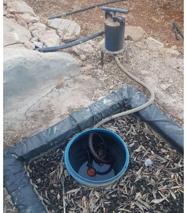
Fig (4): Submerged Pump and Filter
