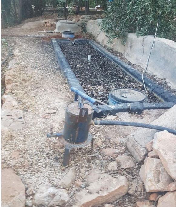
Fig (3): Greywater Station
