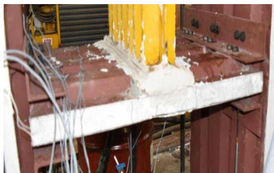
Figure 18: Crack initiation in SFCC floor panel
