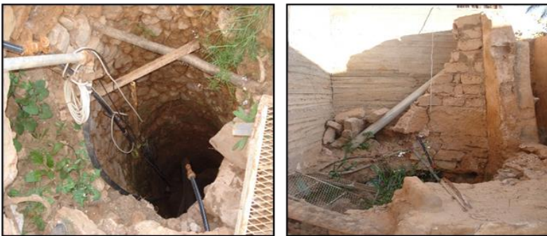
Photo 04: Deterioration of the superstructure and infrastructure of the Boujebouj well in the Qaser Ghardaia oasis.
