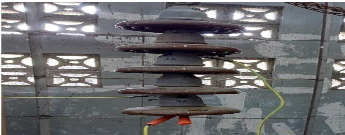
Figure 5. Testing the Breakdown Voltage of the Mossy Insulator
